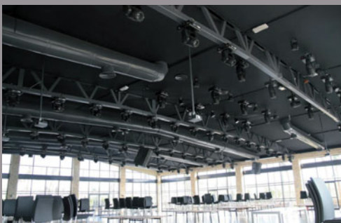
Reception room (Israel) - Installation: Glarus Ltd
